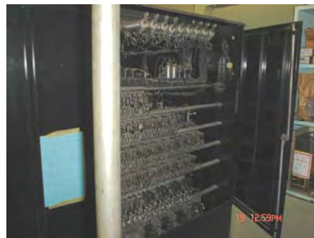
39 Year-Old Elevator Relay Controls
